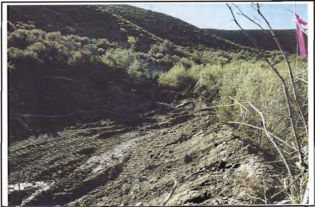
Before: Upstream view of entrance to Channel 10 during construction. Channel 10 is approximately 2000 feet in length.
