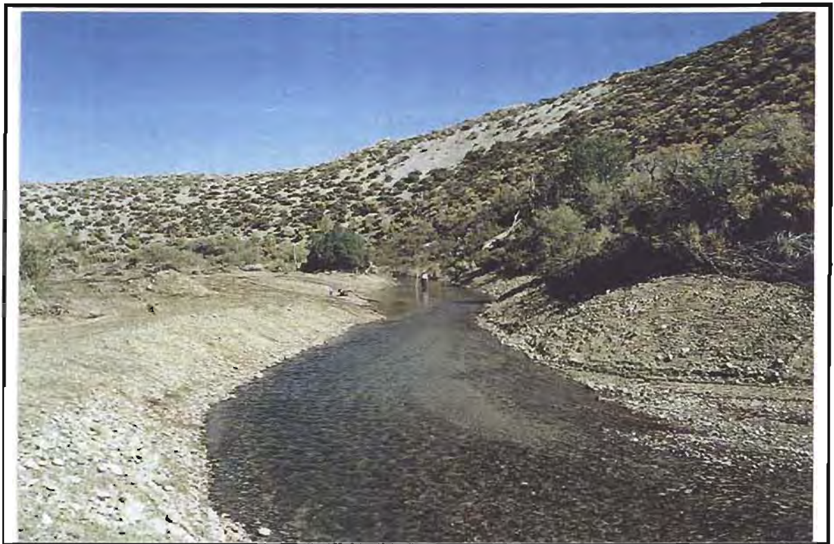
After: View of the constructed channel. Sloping, armored streambanks and point bars were constructed along a planform which followed the toe of the valley wall. After the revegetation of the banks the channel is expected to remain relatively stable through a range of discharges.
