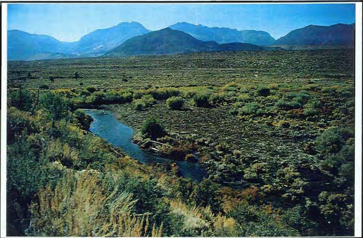
After: View looking upstream along the toe of the valley wall depicting the ~450 ft of constructed Channel 10. ~1500 yds 3 of plug sediments/debris were removed and placed on the adjacent area which impacted ~1 acre of upland sagebrush and rabbitbrush vegetation. The impacted area was seeded with the same native uplandl vegetation. Existing willows were mostly left in tact. Brush was scattered over the area to hold the seeds in place and reduce wind erosion on the site.
