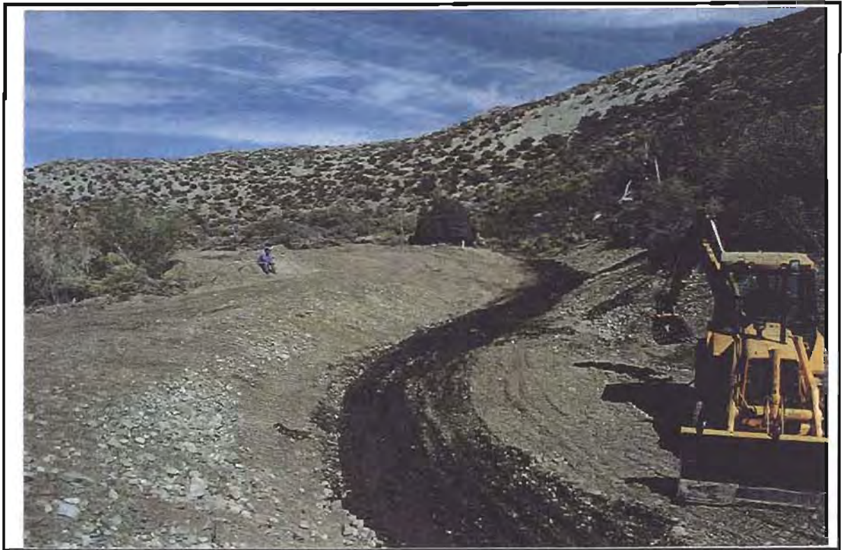
Before: Photograph depicts excavation/construction underway just downstream from the entrance to Channel 10. Removal of the gravel/debris plug took place from the entrance to a point 450 feet downstream.
