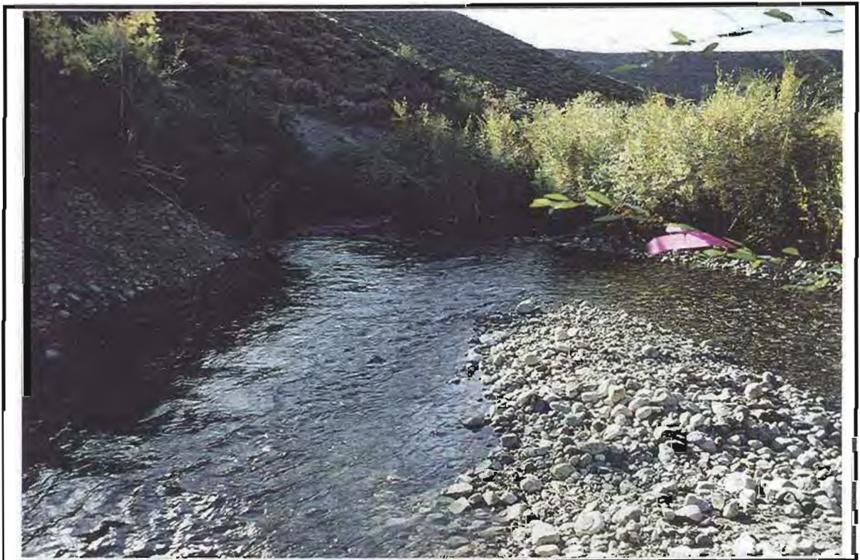
After: Photograph depicts the final configuration of the constructed point bar. The smaller right channel is the existing side channel and the left channel is the constructed Channel 10 entrance. Channel 10 is designed to contain \frac{2}{3} of the incoming flow & the side channel will contain the remaining \frac{1}{3} and function as an overflow channel.
