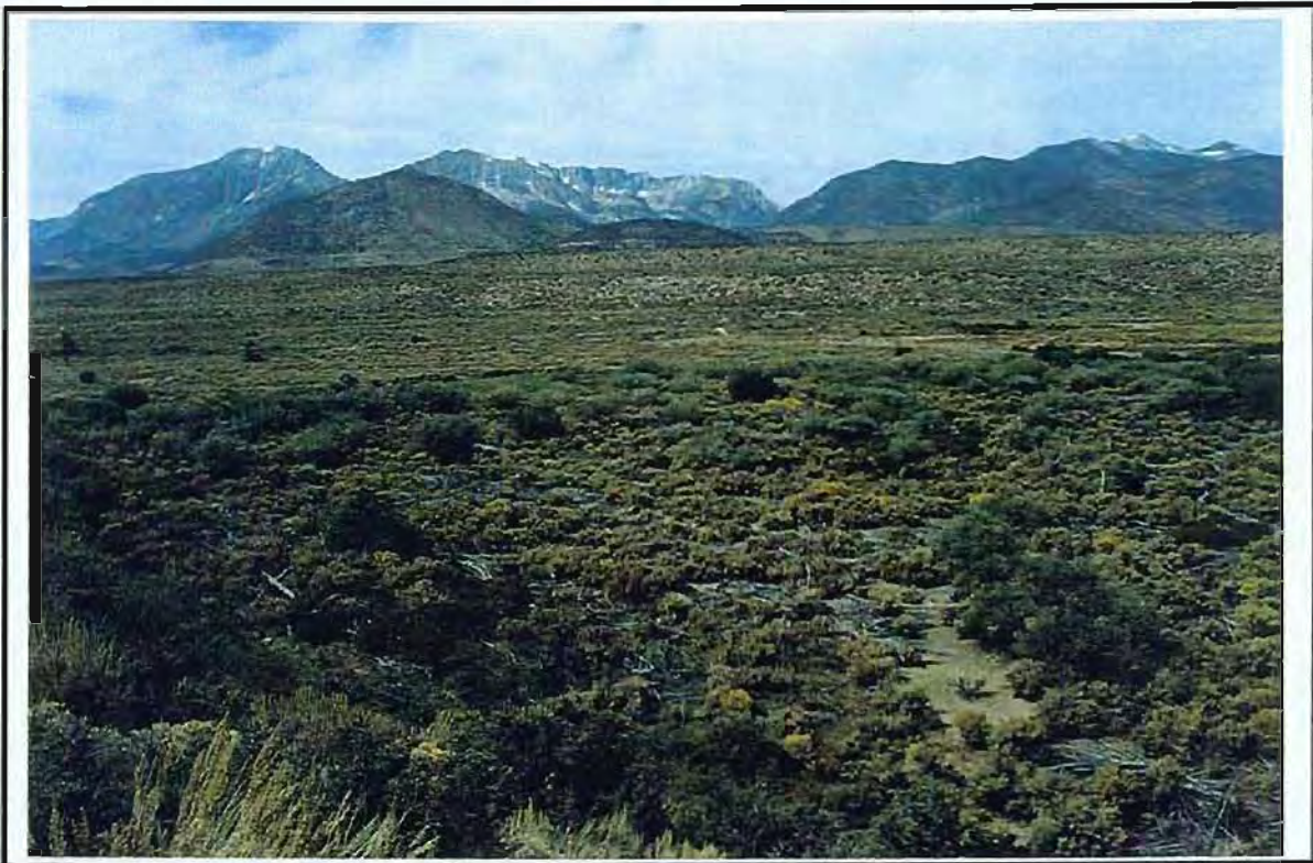
PP4 Before: Upstream view overlooking sediment/debris plug of Channel 10. Approximately 3 to 6 feet of plug materials were excavated & removed from ~450 lineal feet of upper stream channel. Sagebrush and rabbitbrush vegetation was growing over much of the historical channel and adjacent areas.
