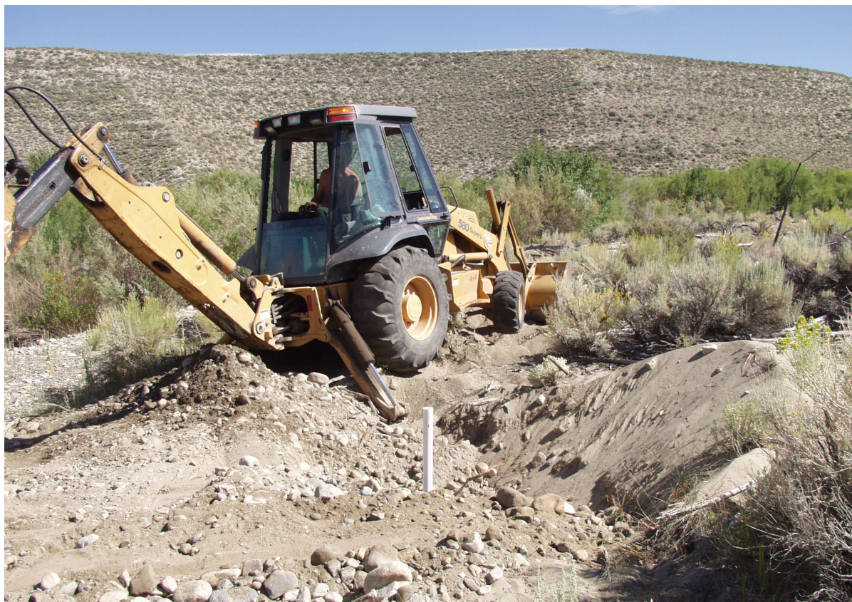
Figure 12. Photograph of a piezometer at the 8-Channel construction site immediately following installation.
